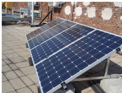
Fig. 9. Four 240 W solar panels as independent energy source
