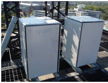
Fig. 7. Two outdoor racks near the antenna tower of primary GND contain power supplies, computers, radio transceivers, power amplifiers, low-noise amplifiers, coaxial relays, resonators as band-pass filter, etc.
