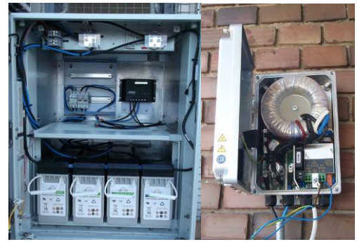
Fig. 10. Four 100 Ah 12 V accumulators with charging controller (left) and the power inverter (right) from 48 V to 230 V, mounted near the solar panels.
